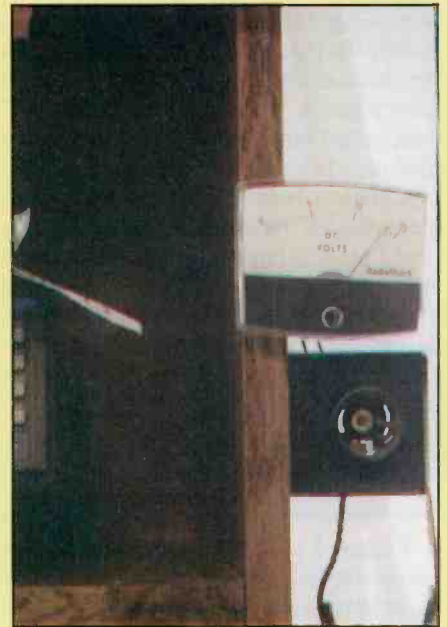
Inside the shack, the meter measures DC voltage and below is one receptacle providing free 12 Vdc power!
