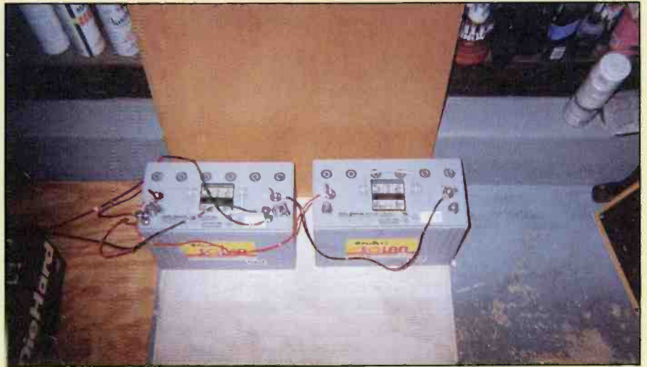
These two Deka batteries are sealed gel cell models and are maintenance-free. Notice the heavy-duty wiring that connects the batteries in parallel.
