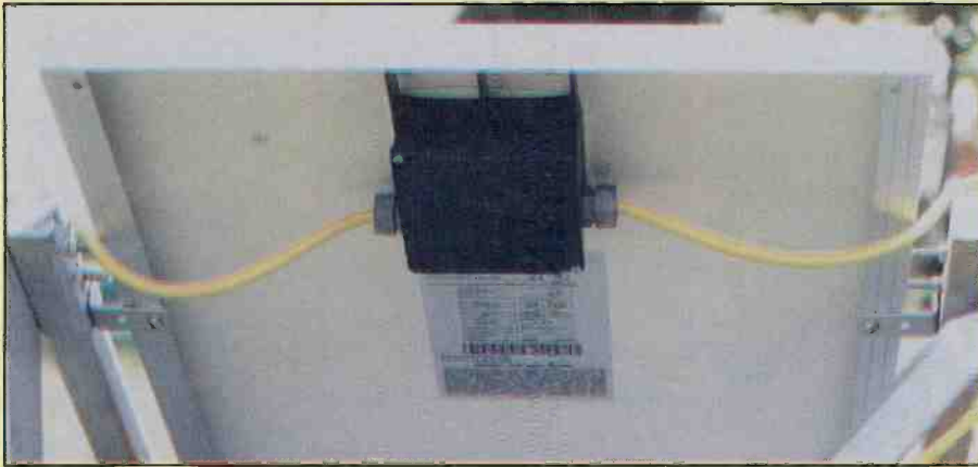
A panel's junction box showing a short outdoor extension cable going to another panel, and the other cable to the charge controller.
