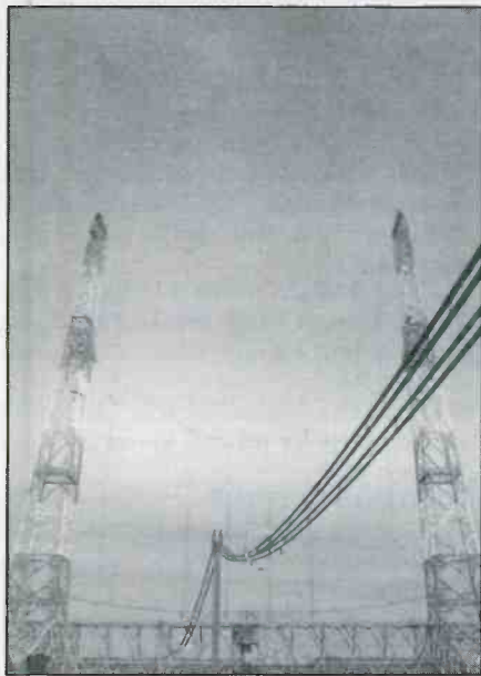
Part of Vatican Radio's antenna system at their Santa Maria de Galeria site in Italy.
