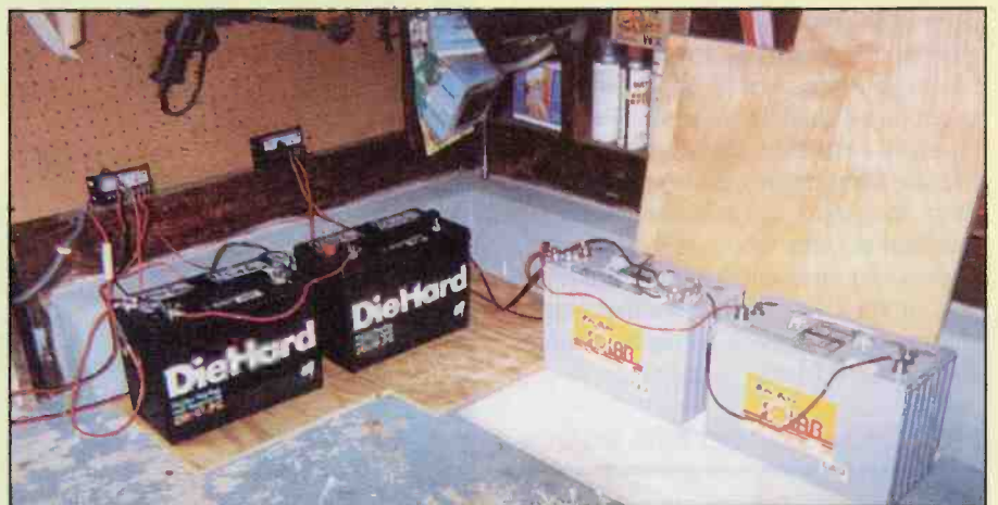
The two Sears DieHard Marine Starting And Deep Cycle batteries and Deka's two high quality state-of-the-art sealed valve regulated (SVR) batteries will provide years of trouble-free service in any small stand-alone solar system.
